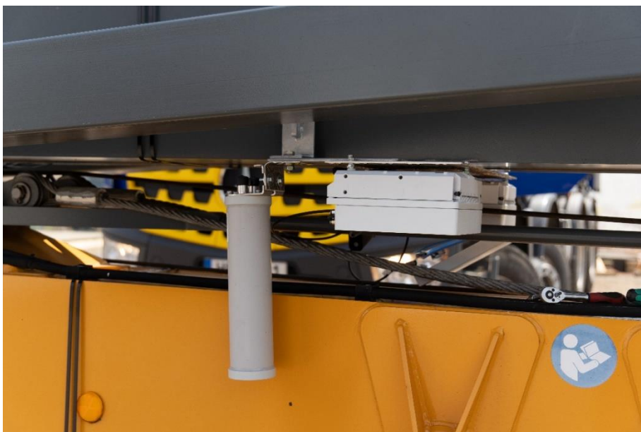
Figure 4.3 5G Antenna and Radio unit mounted to the tower crane.
