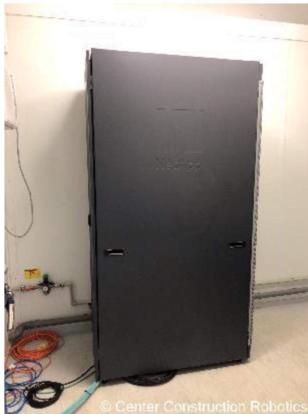
Figure 4: Server room at the Reference Construction Site
