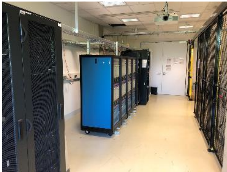
Figure 8: ACS server/real-time lab
