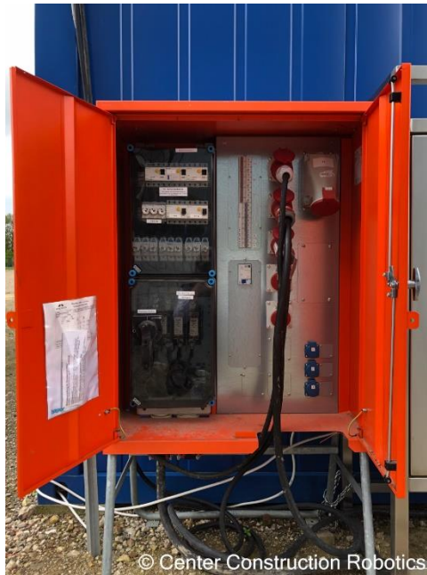
Figure 3: Distribution box at the Reference Construction Site
